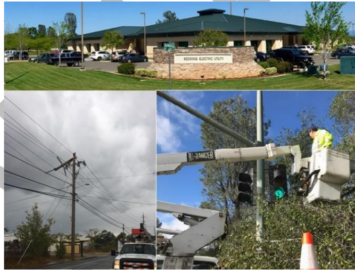
Figure 2. Redding Electric Utility infrastructure
