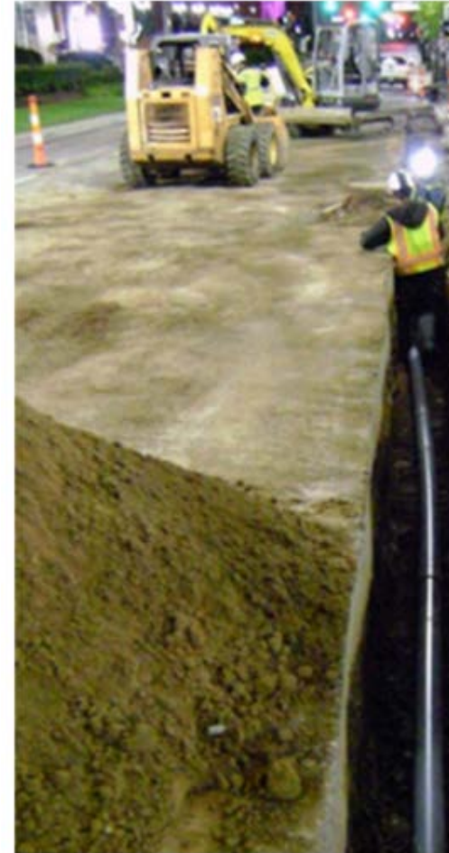
Service ready, high
