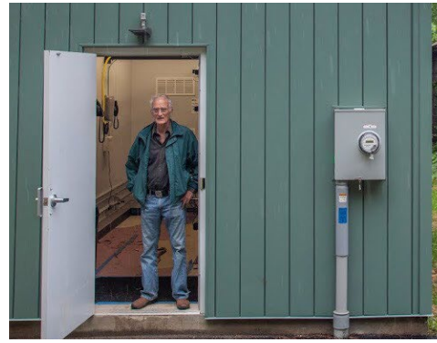
Peter d'Errico, Leverett selectman, in the town's new telecom hut
